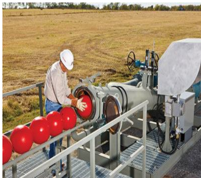
Switching to automated pig launching is one way pipeline operators could save money in an era of low commodity prices. Using equipment that can be remotely programmed to deploy multiple spheres or pigs on a regular schedule could save hundreds of thousands of dollars.
